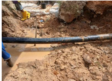
Figure 2. Exposed 6-inch Natural Gas Pipeline in the Excavation at KP.03+500
