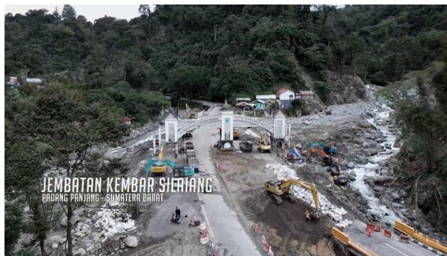
Figure 1. Post-disaster infrastructure recovery around Kembar Sialang Bridge, West Sumatra.
